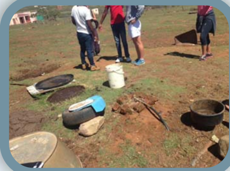
Biogas digester in Macubeni
