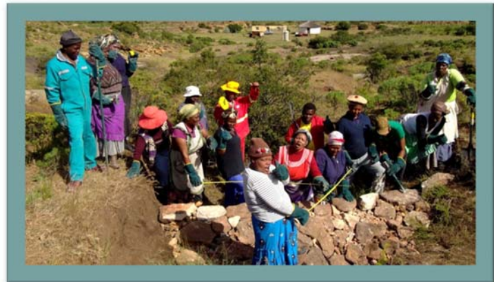
Community members after completing a stone packing exercise to arrest headward gully erosion
