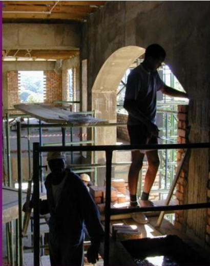
Working on the Hamilton Building to house Computer Science and Information Technology
