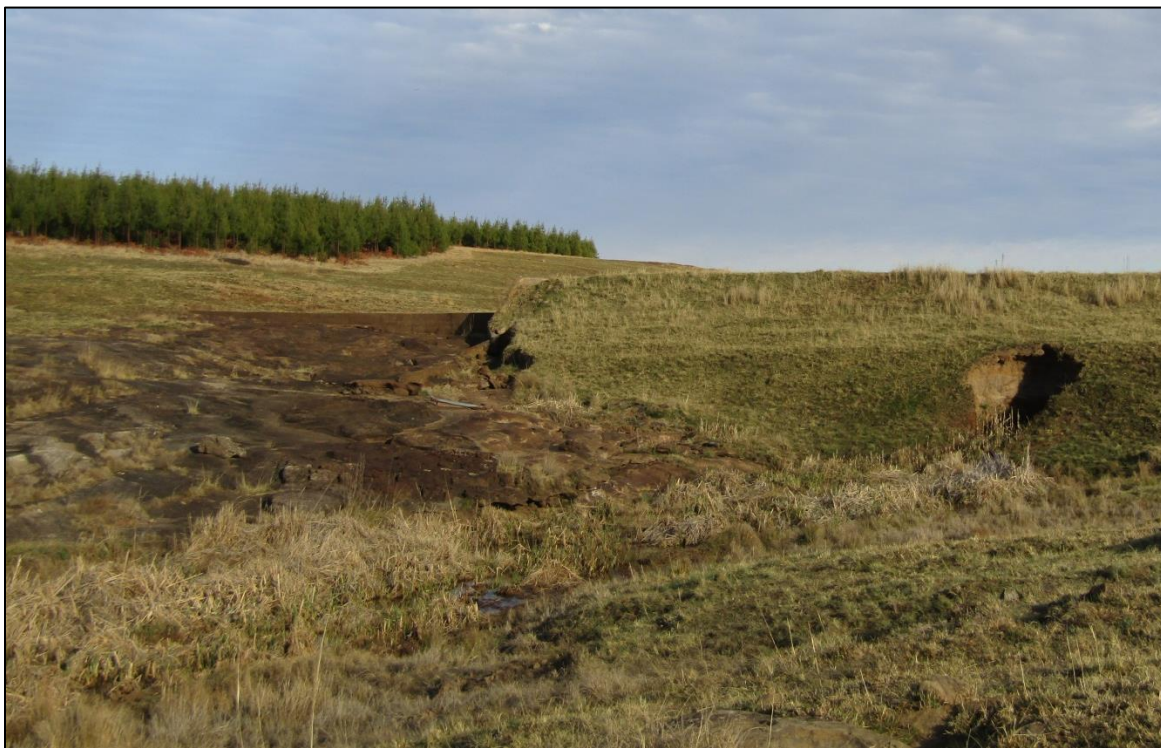
Figure 2: A dam exhibiting an erosional nick point on the dam wall which could result in dam wall breaching
