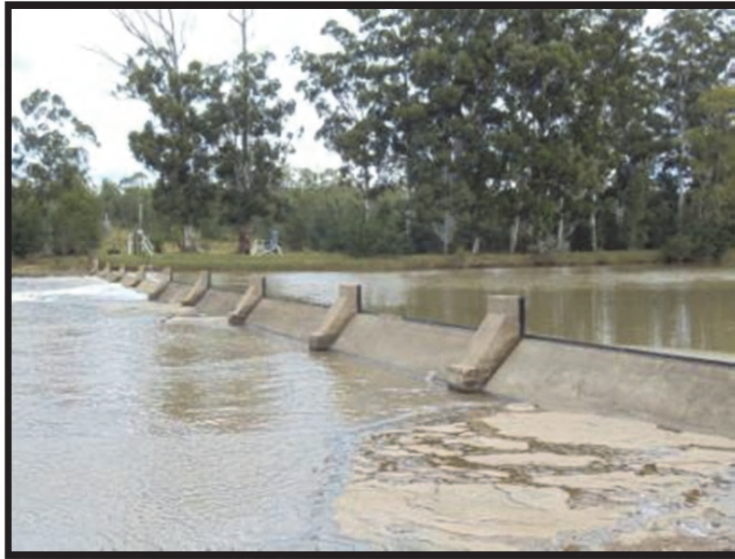
Figure 2.10: DWA gauging weir T3H006 approximately 20 km downstream of the proposed dam wall (Photo 1 in Figure 2.2).
